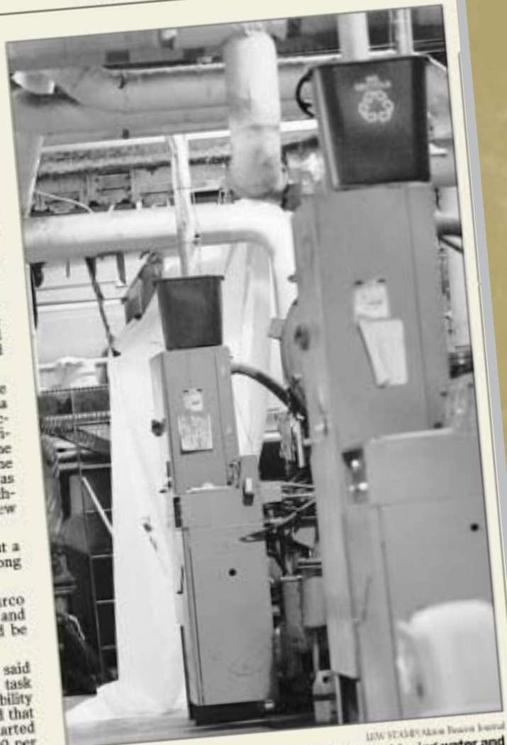
Waste baskets atop electrical equipment collect dripping water and white plastic sheets cover communications equipment on the 10th floor of the Harold K. Stubbs Justice Center.
